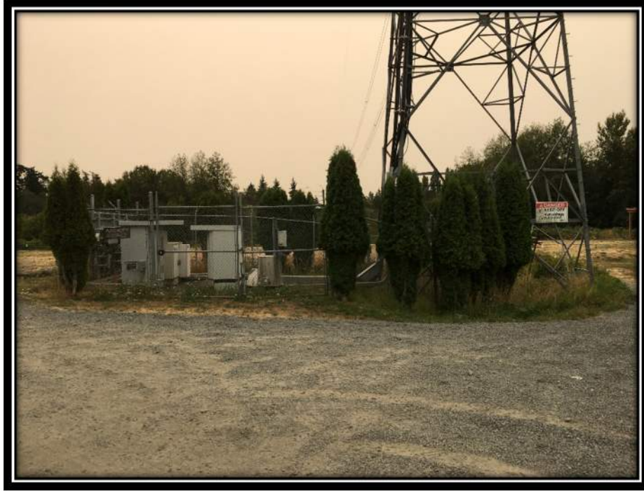
Photograph 5: Photo showing the base of the BC Hydro Electrical Transmission Tower (APEC #4). Photo looking southeast.
