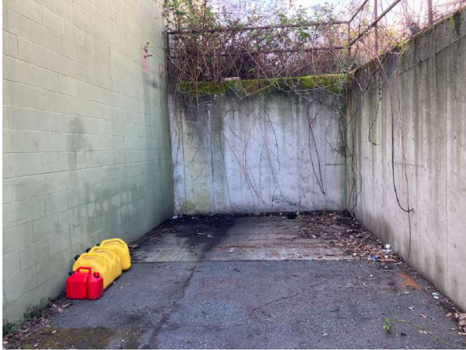
Photograph No.5: View of staining on concrete on the western side of the building.
